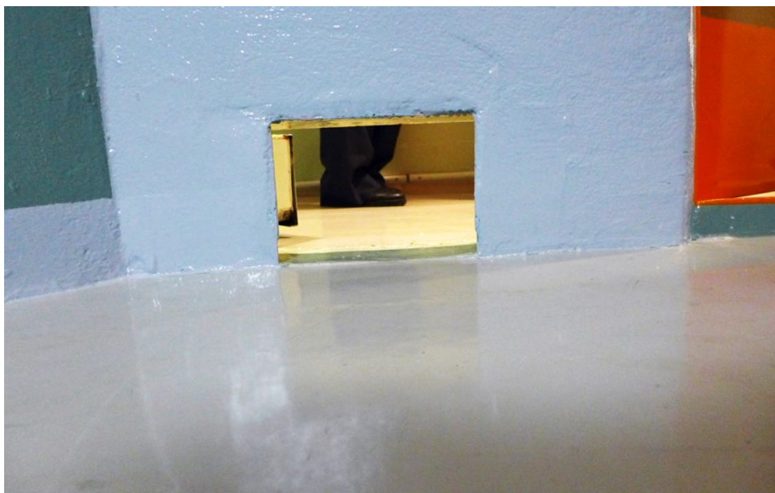
Hatch at floor level for delivering food to persons in security cells. Telemark prison, Skien unit. Photo: The Parliamentary Ombud.
